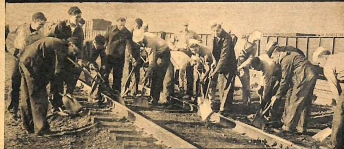
NAVY HELP. Sailors from the Norfolk (Va.) Naval Training Station pitch in during a shortage of manpower by working on the tracks near Norfolk.
