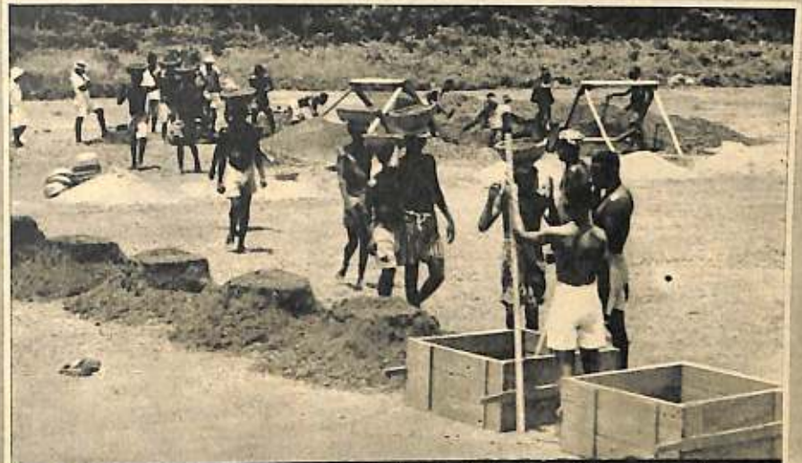
African nudies, who are a set of nicely balanced boys, are busy building a runway at a new West African airfield. It's a stopping-place for Middle East-bound aircraft.
