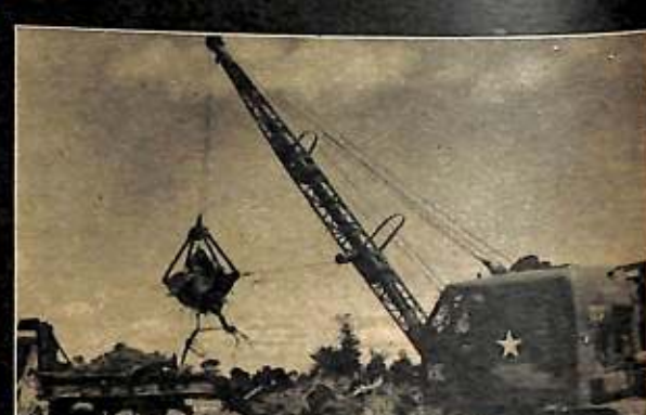
3 NEXT, A CLAMSHELL STEAM SHOVEL SWIFTLY CLEARS AWAY TREES AND HEDGES TOPPLED BY THE 'DOZERS.
