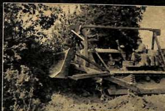
2 THESE NORMANDY HEDGEROWS, IMPLACABLE FOE OF ADVANCING TROOPS, ARE NO MATCH FOR A BULLDOZER.
