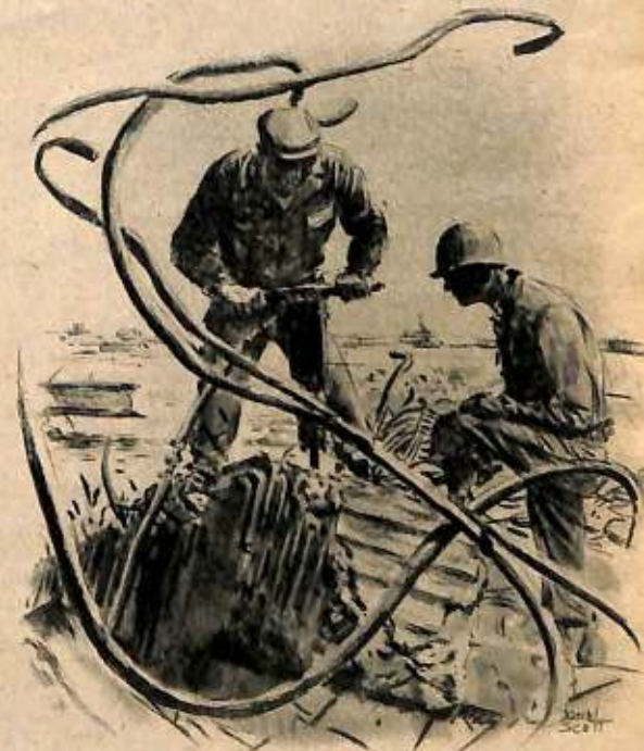
CPL. RICHARD W. FITZ OF COMPTON, CALIF., DRILLING HOLES FOR BLASTING CHARGES AMONG THE TWISTED STEEL OF REINFORCED CONCRETE ON THE TRANSATLANTIC QUAY.
