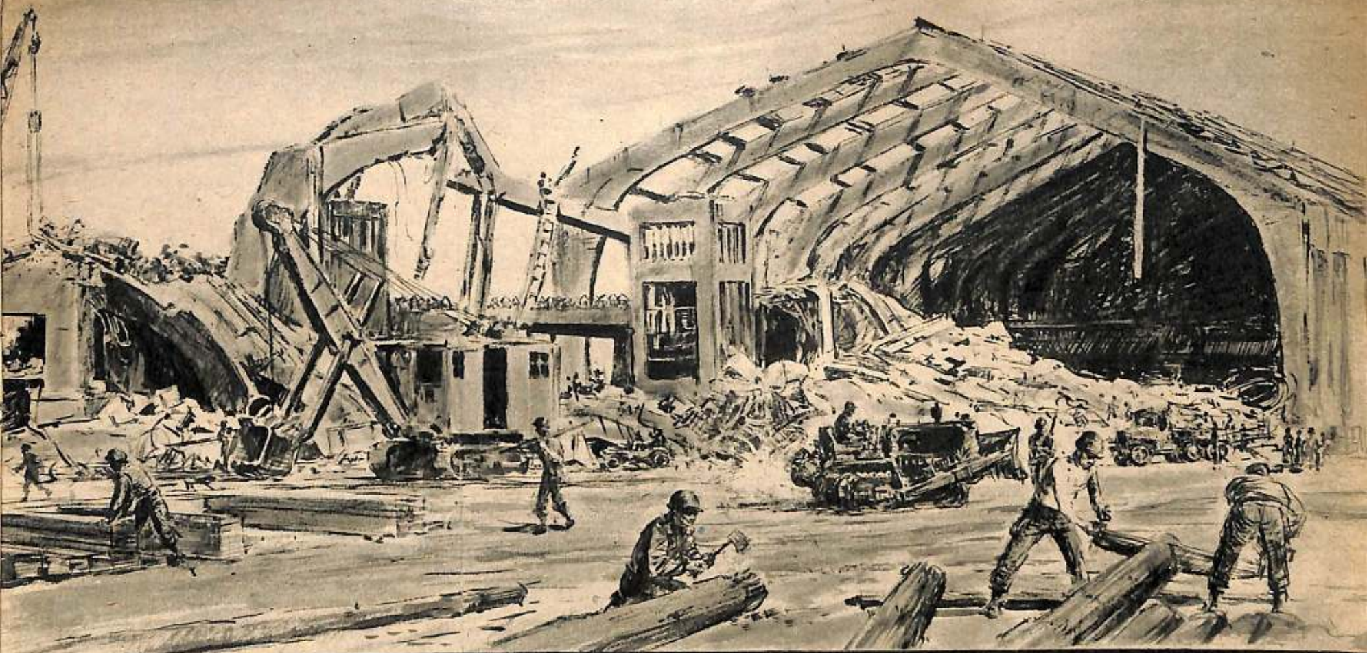
TWISTED WRECKAGE OF THE GARE MARITIME ON THE TRANSATLANTIC QUAY AT CHERBOURG. BEFORE THE WAR, LUXURY LINERS FROM NEW YORK DOCKED HERE AND PASSENGERS COULD WALK DIRECTLY ABOARD A PARIS-BOUND TRAIN. THIS QUAY WAS CHOSEN FOR THE MOST COMPLETE DEMOLITION BY THE GERMANS BEFORE THEY SURRENDERED THE PORT—AND THE NAZIS SUCCEEDED. ENGINEERS ARE PLOUGHING INTO THE DEBRIS WITH BULLDOZERS, REMOVING THE RUBBLE AND REBUILDING THE ESSENTIAL PARTS.
