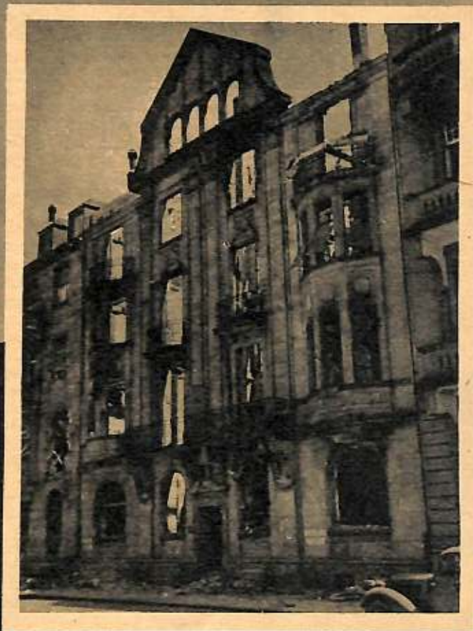
Walter's home - where, you remember, we used to have parties; a sign says "Danger of Collapsing"
