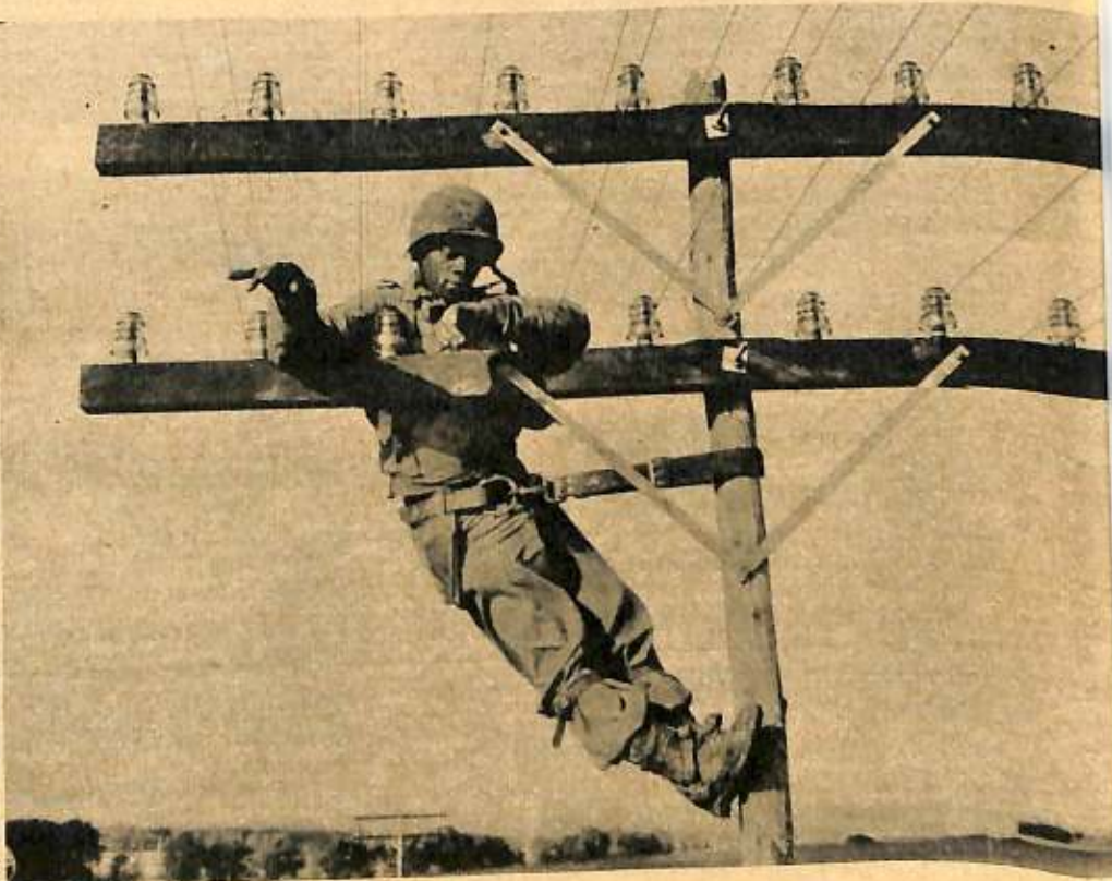
TUNING. Pvt. Russell Myers of the Signal Corps is checking line sag on this pole in France, using the oscillation method for proper wire tension.
