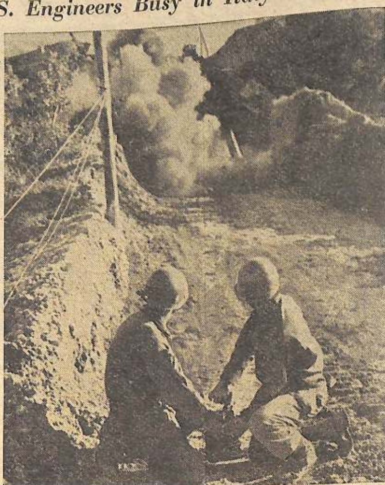
A dynamite charge clears away Nazi-sown obstructions on a road to be repaired in western Italy. Road repair is a breeze, Engineers claim, constructing pontoon bridges across wild Italian rivers are the real headaches.
