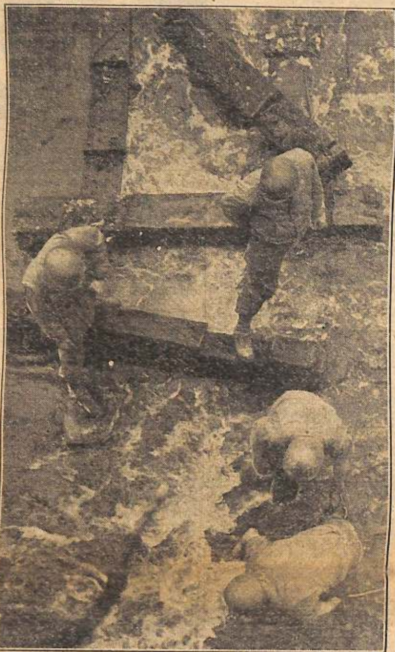
A stream is clogged with debris of a bridge which retreating Germans had blown up near Spa, Belgium. The stream has to be cleared quickly, so the engineers get at it. This Signal Corps picture shows how they remove bridge girders from the swift-running waters.
